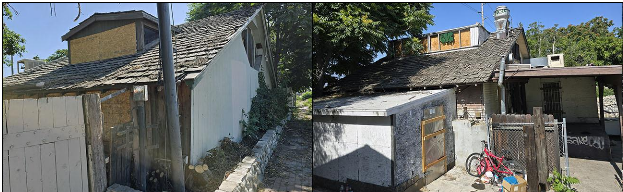
Building C, restaurant/bar. Left: front and eastern façades, view to the southwest; right: refrigeration room and rear patio, view to the east
